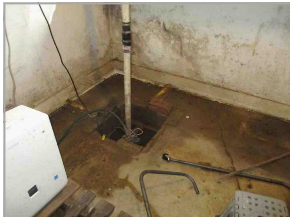
Basement Water noted
