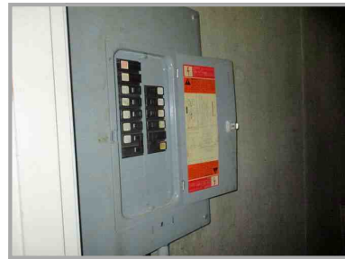
Electrical Service Panel
