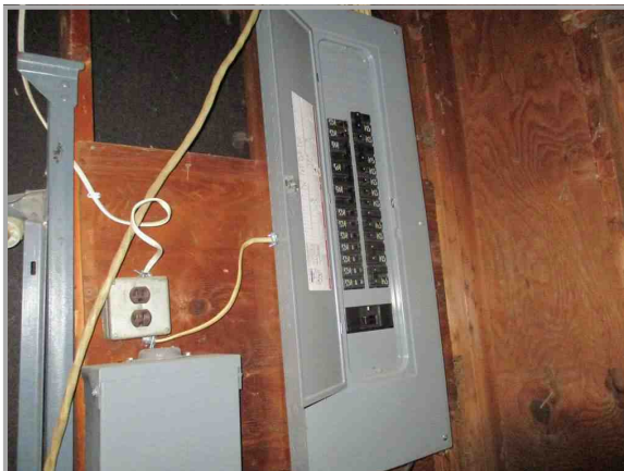
Electrical Service Panel
